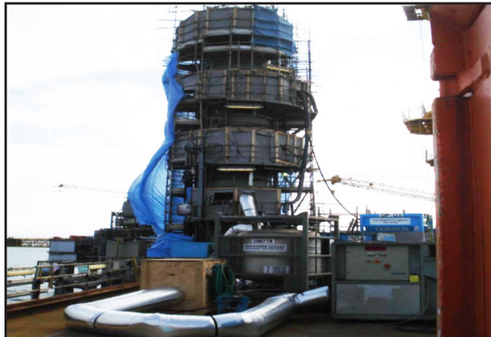
Deaerator on offshore platform
